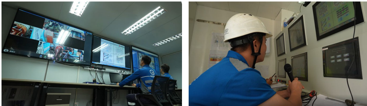
Figure 24 - Central Monitoring Station (left) and Operator Cabin in Site Control Room (right)
